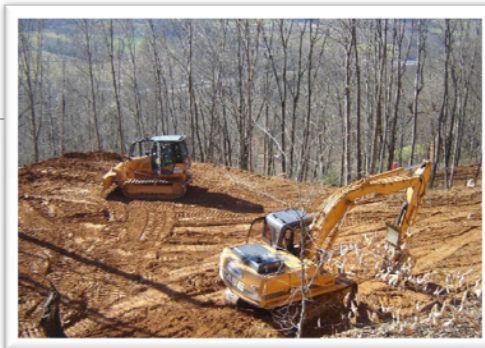
Areas that are disturbed during grading (above) are prone to soil erosion and compaction.
