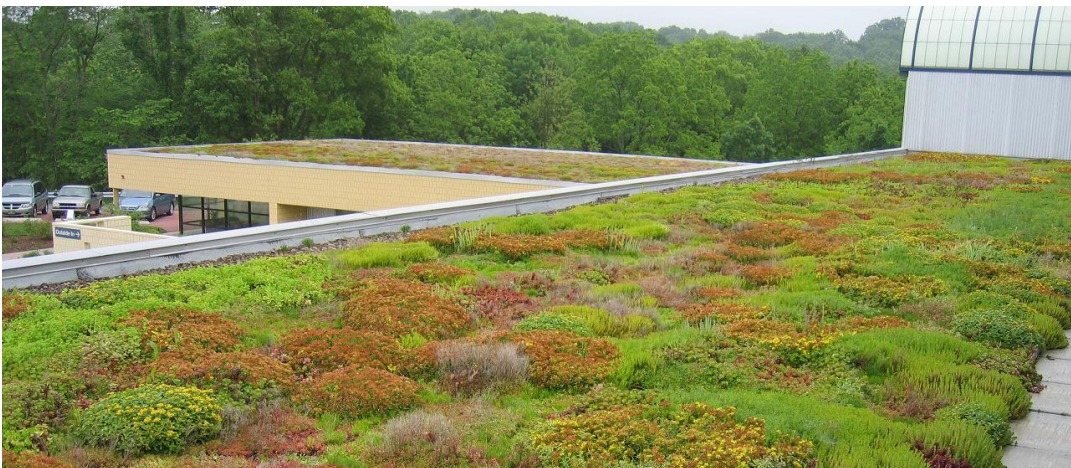
This vegetated roof in Westmoreland County is located at the County Conservation District's office. This installation was part of extensive sustainable stormwater retrofit solutions across the site. Photo: wcdpa.com
