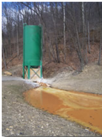
Figure 7. The Lucerne 3A Limestone Dosing Silo.
