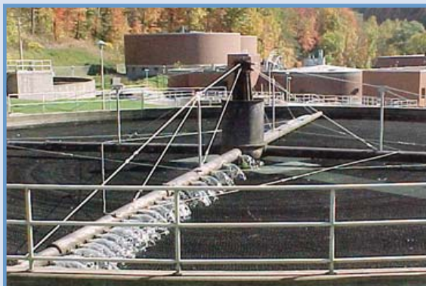
Franklin Township (Murrysville, PA) Wastewater Treatment Plant. Foreground is media trickling filter, background is nitrification towers (left) and sludge digesters (right).
